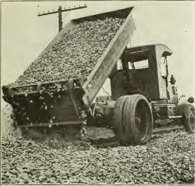
Auto truck used in putting rock on the J. H. in Bourbon County, Kansas.
