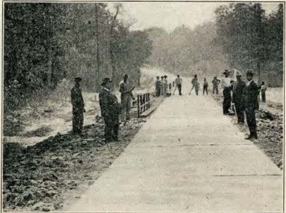
2,000 Lineal Feet of Concrete Road on the Jefferson Highway in Camp County, Texas, Across Cypress Bottom.
