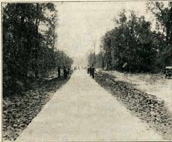
One mile of concrete road on Jefferson Highway in Camp County, Texas, near Pittsburg, Texas.
