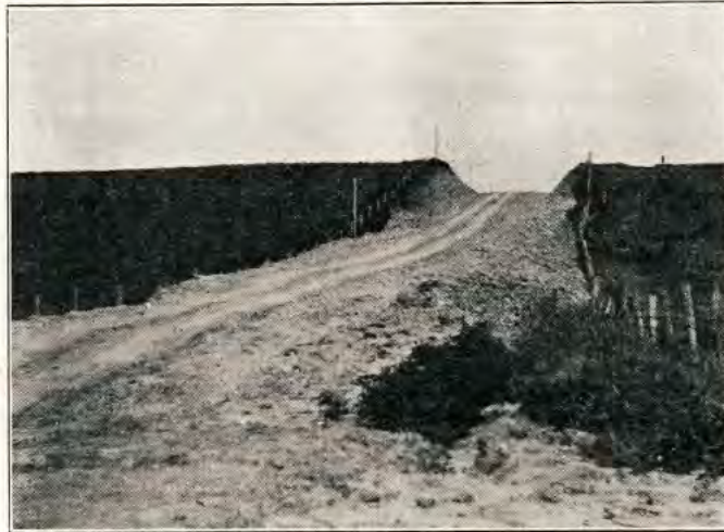
Recent cut made in hill on the Bethany and New Hampton, Missouri road.— A section of Jefferson Highway
